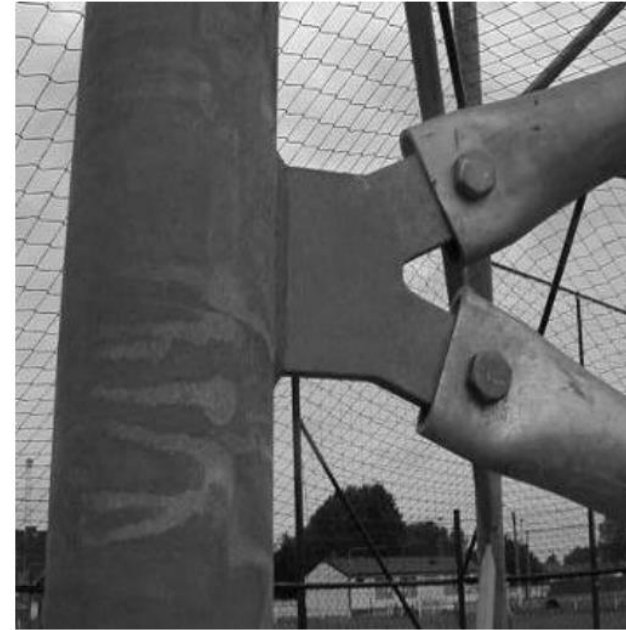
Figure 11: New joint between diagonal and leg, both circular tubes. KPN-Orange in Belgium
